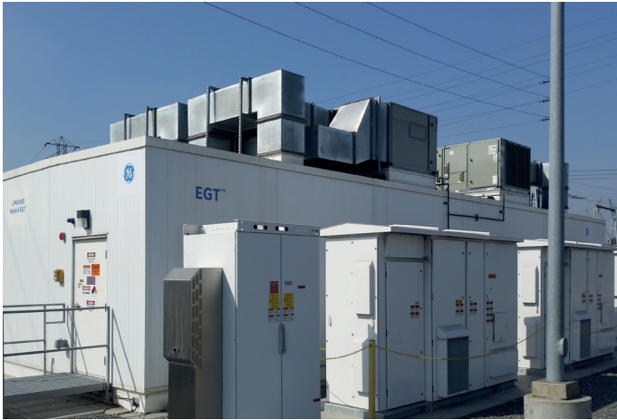
Battery Energy Storage System (BESS)
